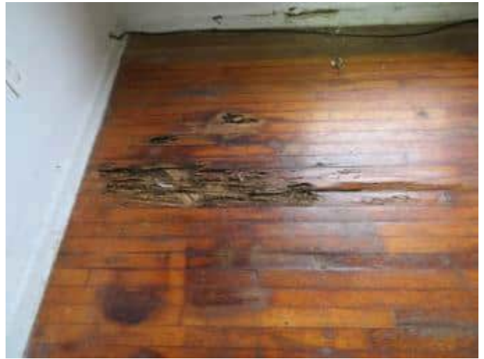
105. Distressed wood flooring.
