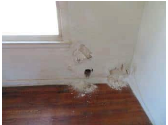
95. Typical distressed finishes at dwelling unit.
