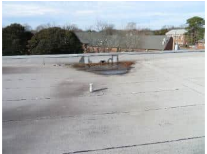
51. Possible ponding around roof drain.
