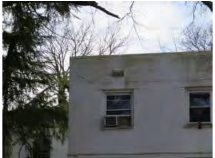
29. Cracking brick at upper portion of the building.
