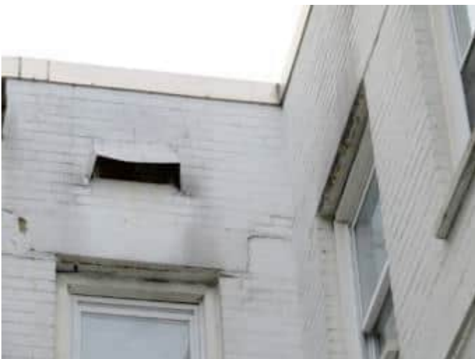
36. Cracking and possible off-plane movement at concrete over window.
