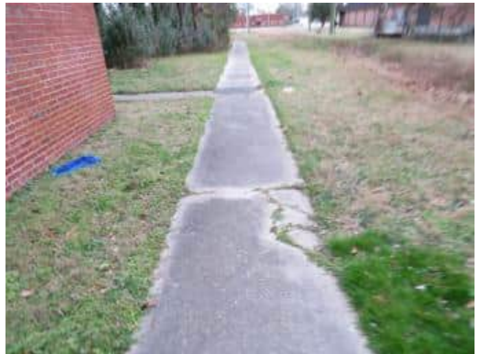
17. Area of concrete flatwork distress at parking garage areas.
