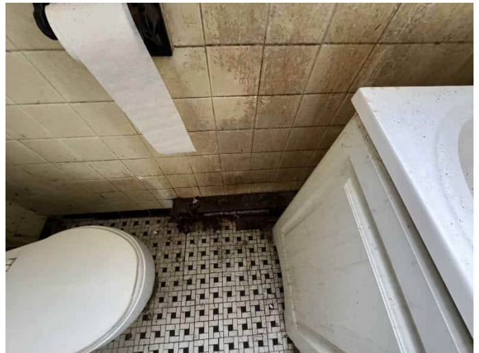
71. Bathroom baseboard heater.
