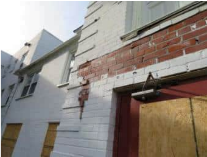
38. Blistered and peeling paint at exterior.
