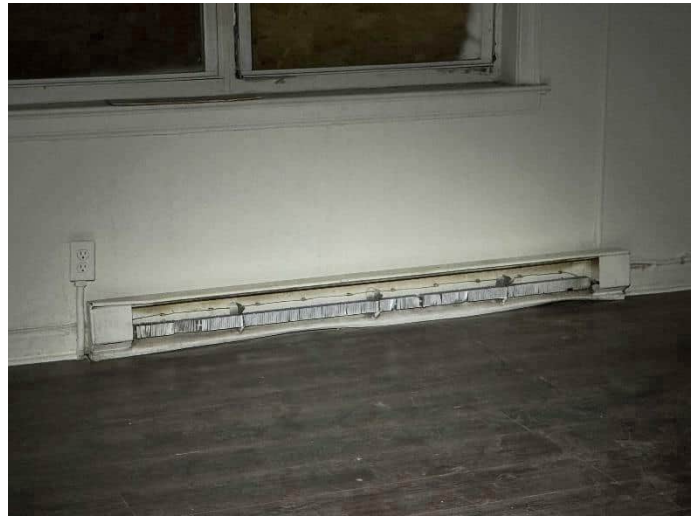
69. Living room electric baseboard heater.
