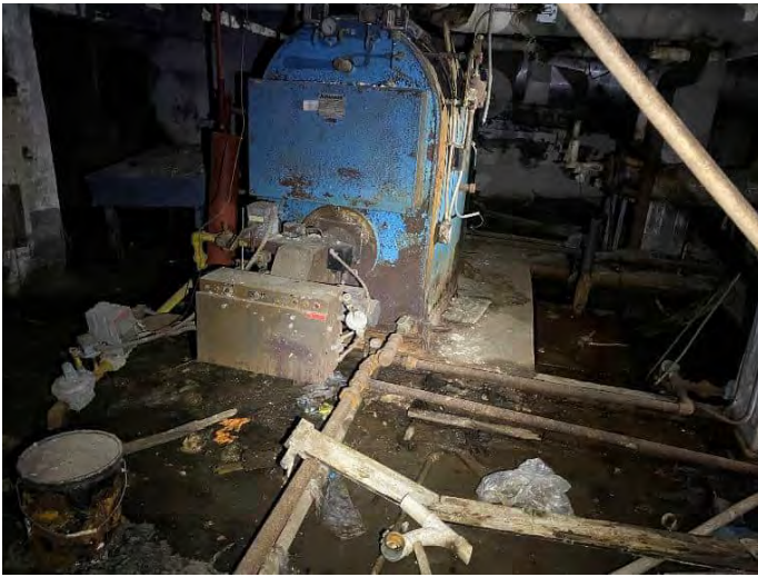
110. Debris on the basement floor interfering with drainage to sumps and standing water in sumps.
