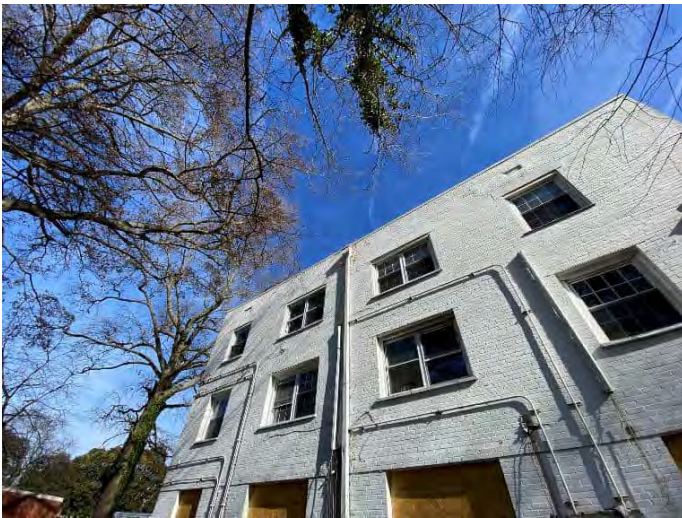
112. Stair-step cracks in exterior brick, typically begin at the upper corner of window openings.
