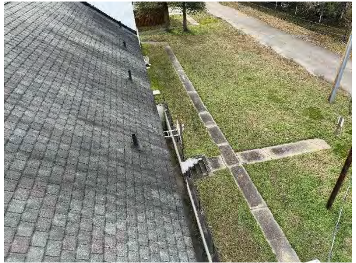
57. Cast iron sanitary vents.
