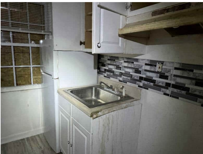
60. Residential kitchen faucet and sink.
