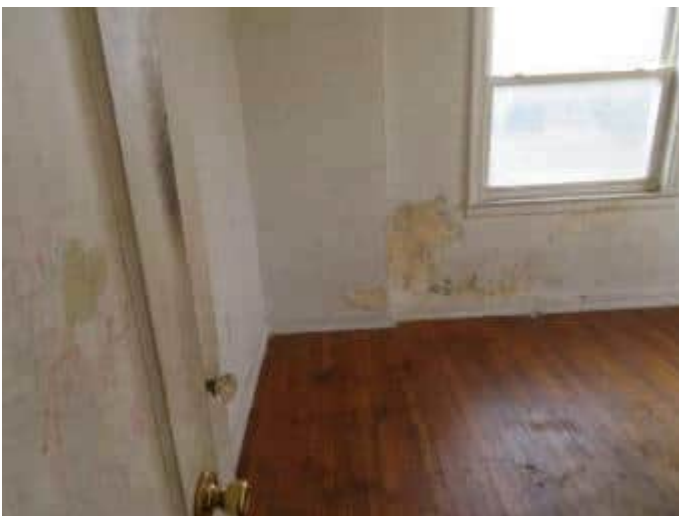
102. Typical distressed finishes at dwelling unit.
