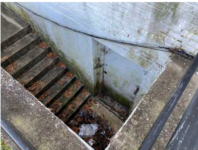
108. Significant accumulation of debris in exterior stairwells leading to basement at Building 2111.
