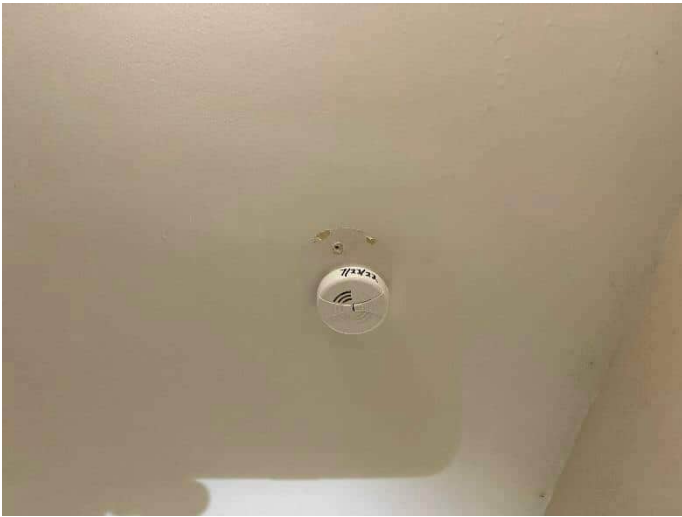
86. Common area corridor smoke detector.
