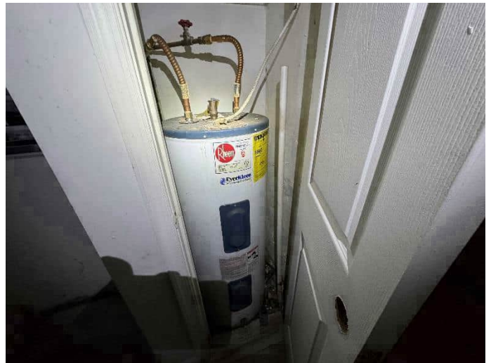
59. Residential DHW heater and copper piping.
