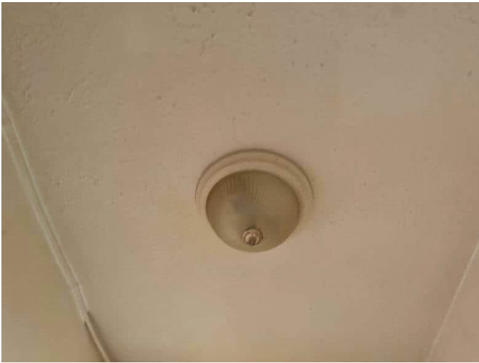
80. Residential hallway lighting fixture.
