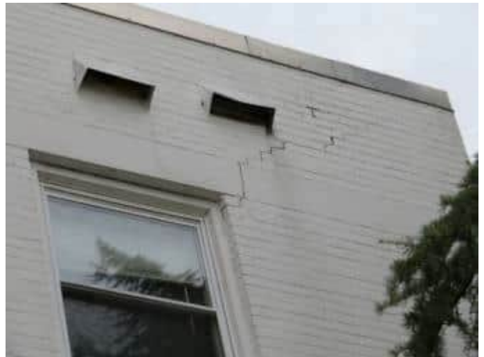
35. Cracking brick and concrete at building upper level.
