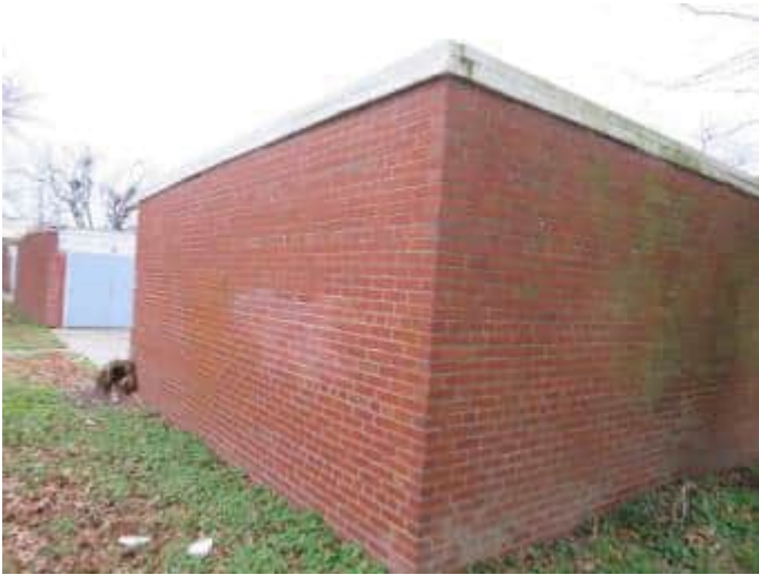
8. Staining at exterior of garage building.
