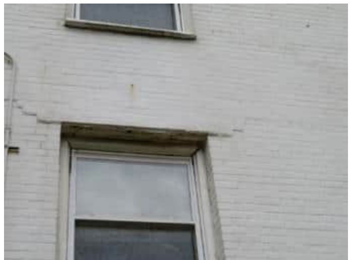
37. Cracking and possible off-plane movement over window.
