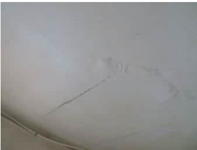
96. Water-damaged ceiling finishes at dwelling unit.
