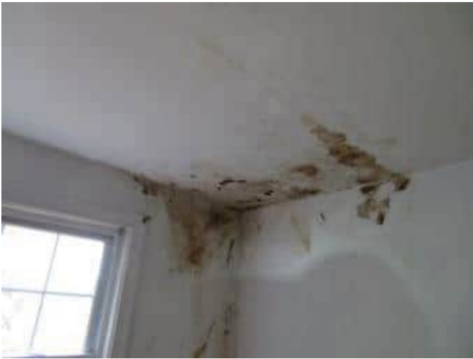
104. Water-damaged ceiling finishes and possible microbial growth.
