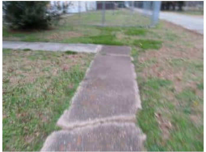
15. Localized cracking and distressed concrete flatwork at the site.
