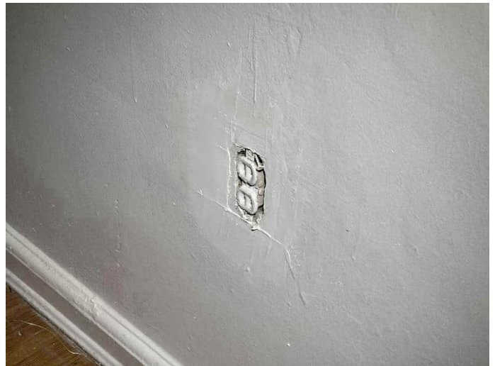
83. Missing electrical outlet cover.
