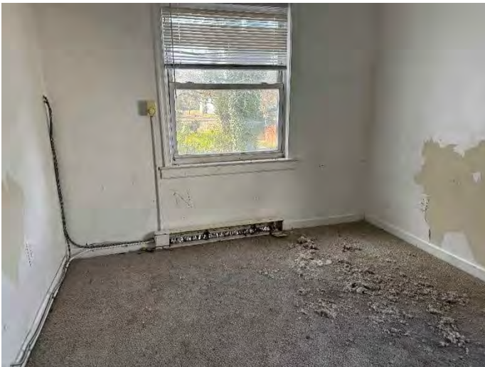
70. Bedroom baseboard heater.
