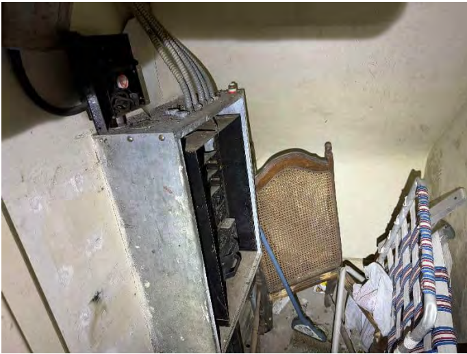
74. Typical building distribution panel.
