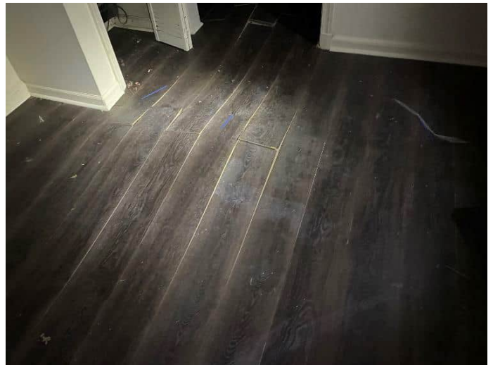
113. Finish flooring in many units exhibit areas where flooring is uneven or buckled and arching upward.
