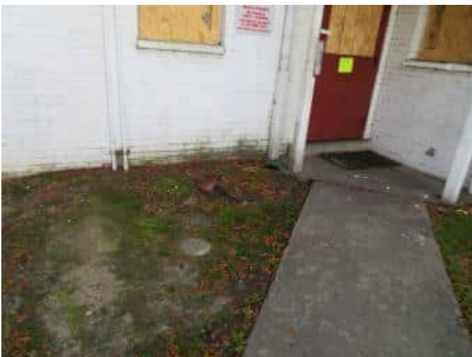
18. Localized area of barren soil at building perimeter.
