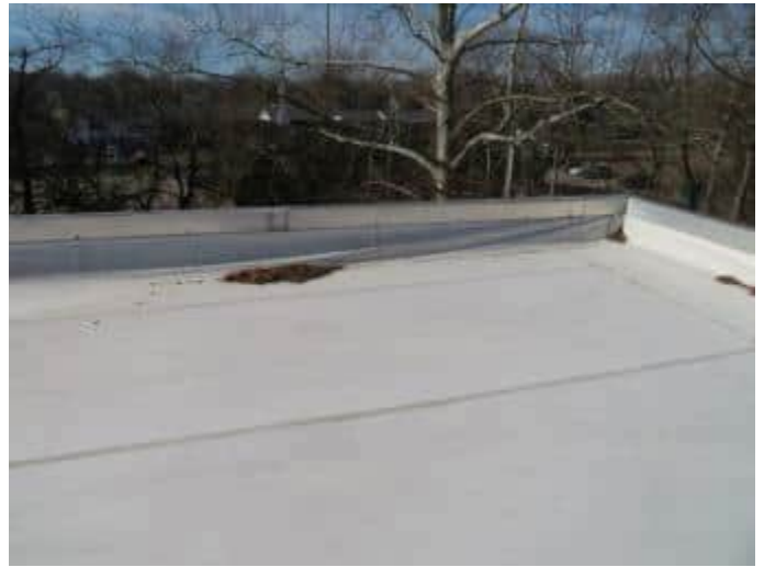
45. Loose membrane along parapet wall and vegetative debris.
