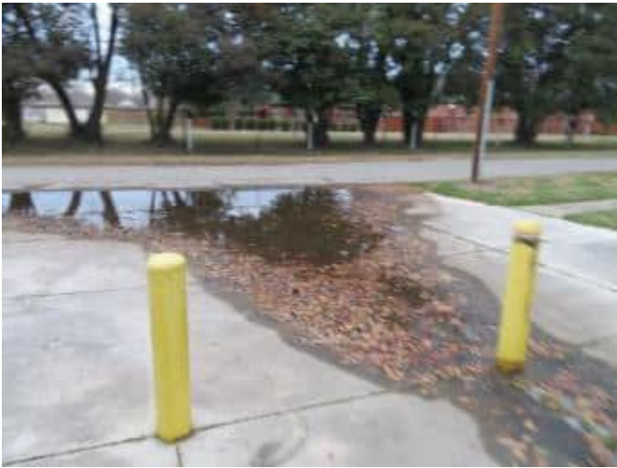
14. Localized depressed concrete pavement at the site.
