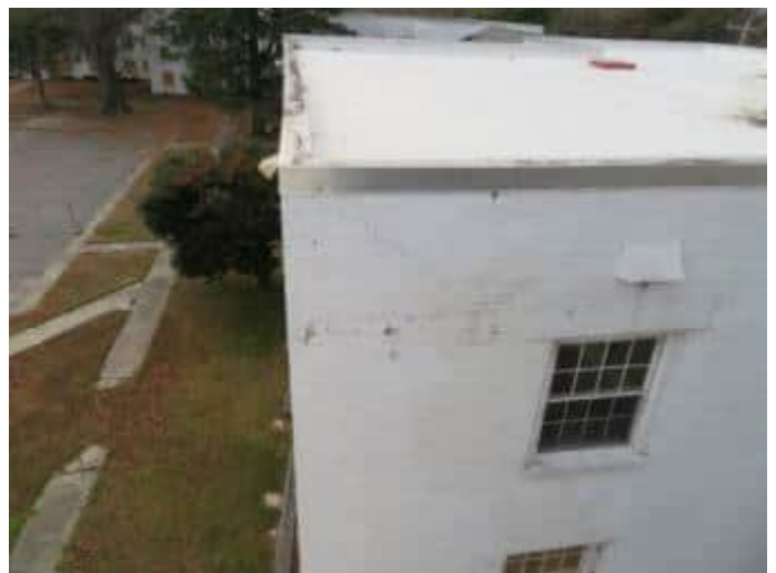
31. Cracking at upper portion of building.
