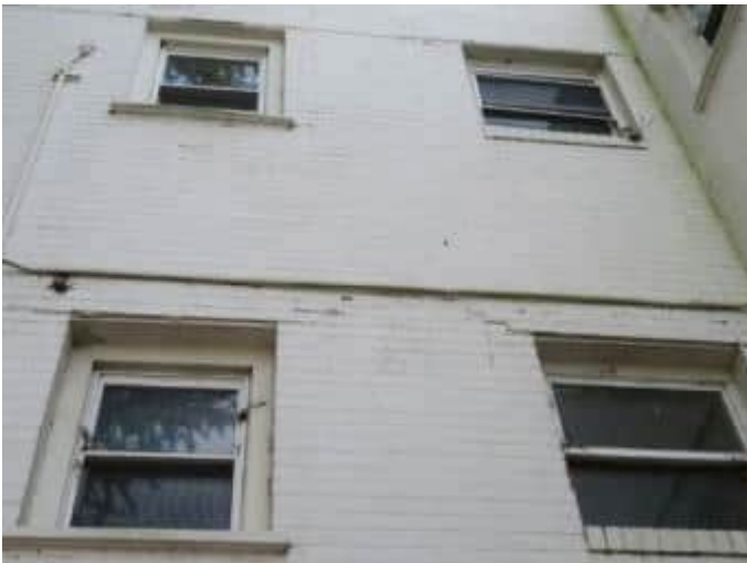
28. Localized step cracking and possible off-plane movement at masonry over window.
