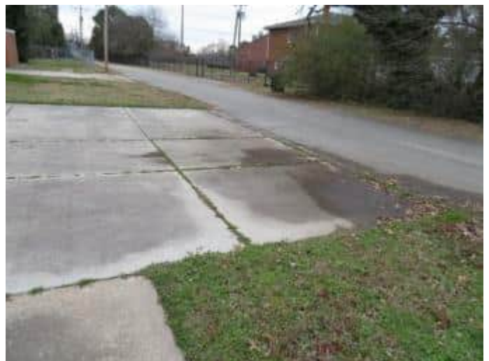
13. Localized distressed concrete pavement at parking garages.
