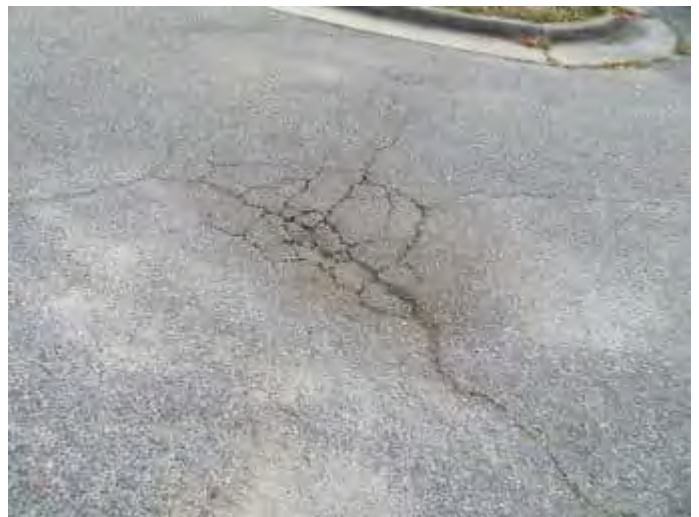
4. Localized asphalt pavement distress.
