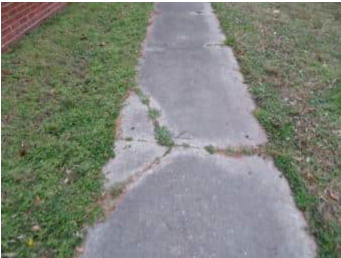
16. Distressed concrete flatwork at the site.
