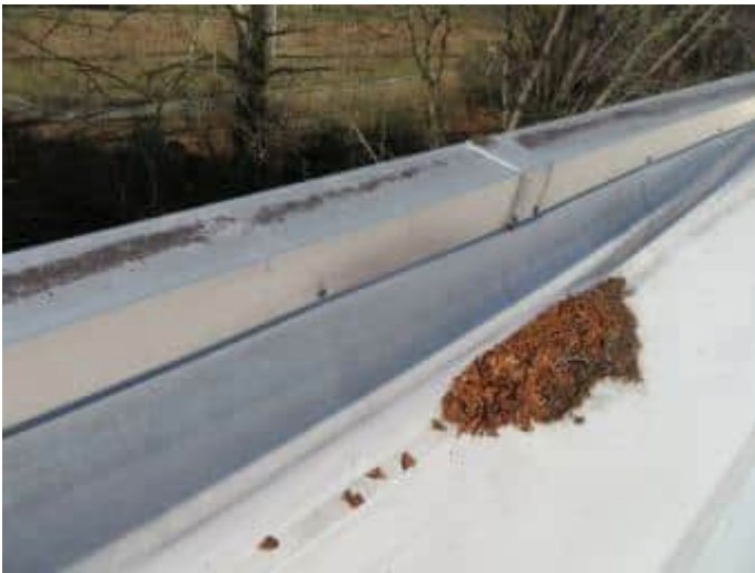
46. Vegetative debris at parapet wall.
