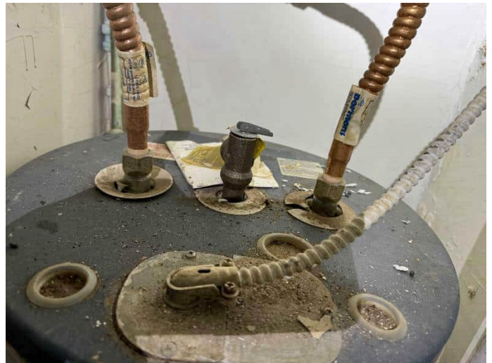
65. DHW heater missing safety release valve piping.
