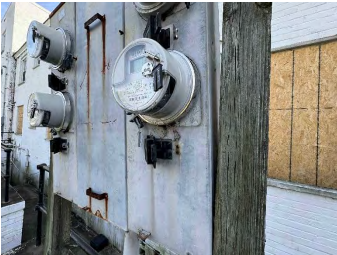
76. Residential meters with main breakers.
