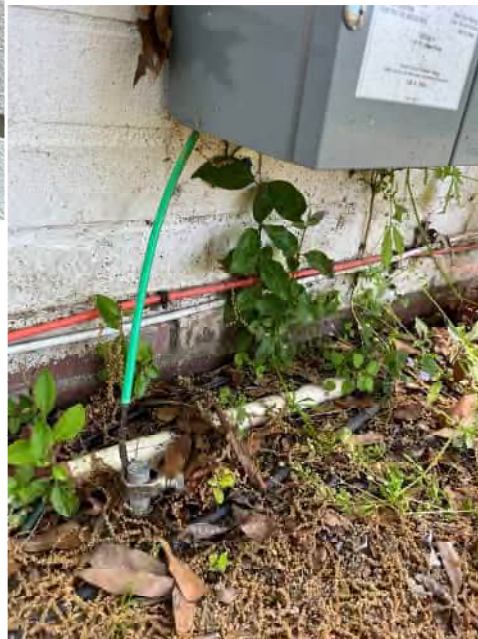
(New meter bank with grounding for reference)
