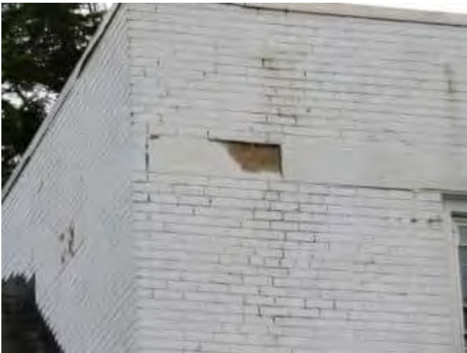
40. Spalling concrete at exterior.
