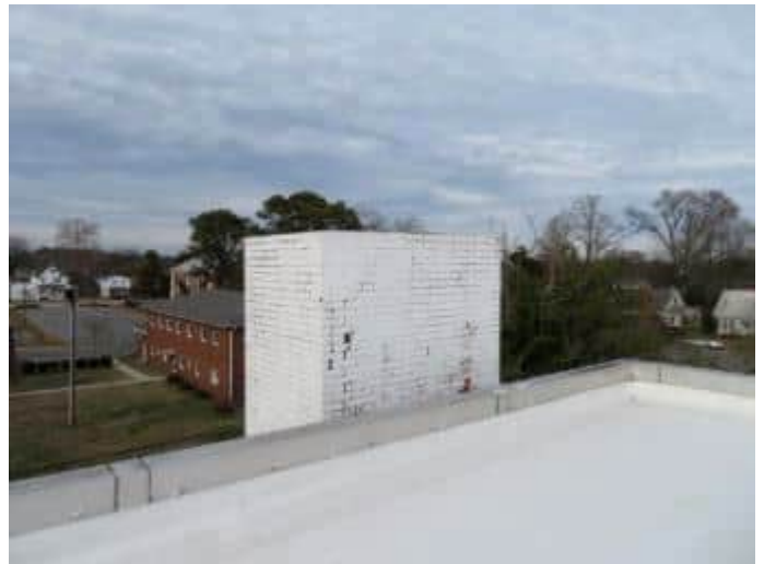
41. Localized step cracking at brick chimney.
