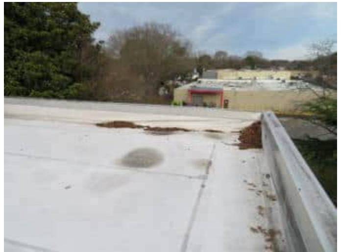
47. Vegetative debris and loose membrane.
