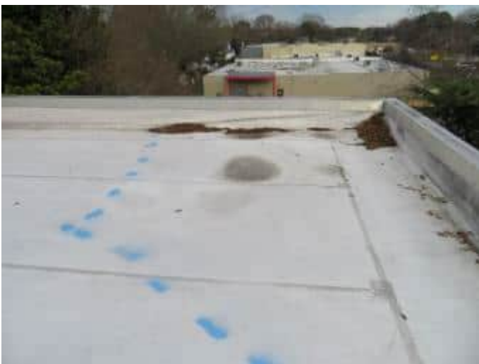
48. Area of possibly damaged roof structure at Building 2115.
