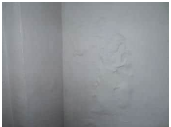
97. Water-damaged wall finishes at dwelling unit.
