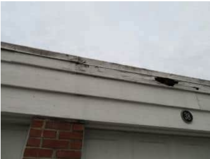
10. Distressed wood at garage exterior.
