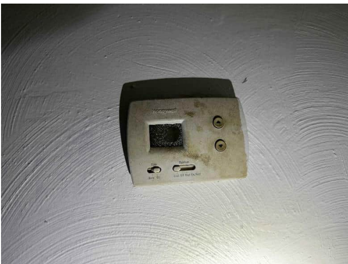
72. Thermostat controlling split system.
