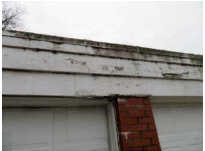
9. Distressed wood and staining at garage exterior.
