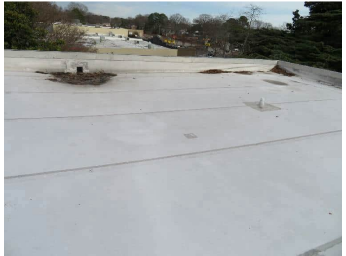
111. The roof surface deflects noticeably in the vicinity of the easternmost corner of Building 2115.
