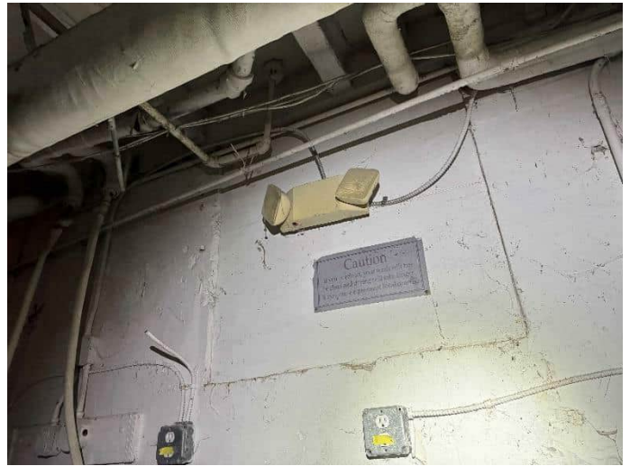
87. Emergency lighting fixture.
