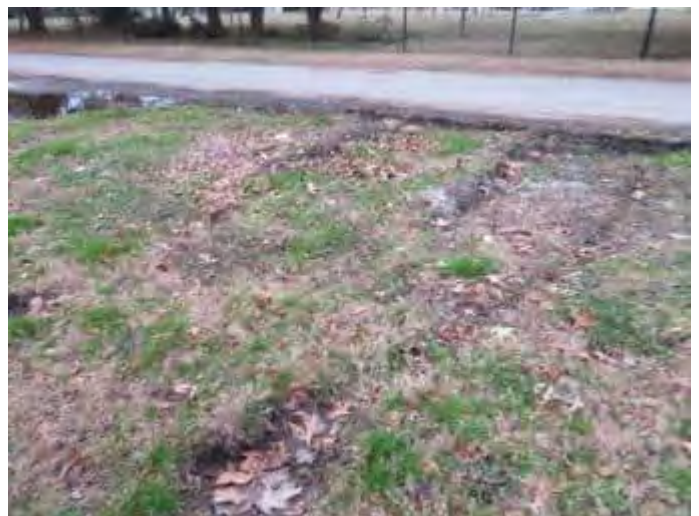
19. Localized erosion at the site.
