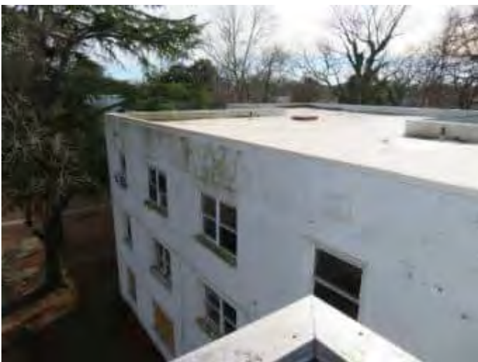
30. Staining at building exterior.
