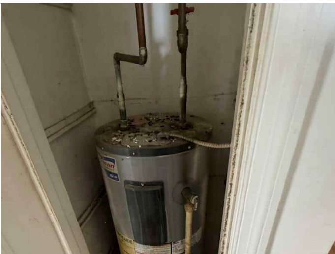
54. Copper piping and electric domestic water heater.
