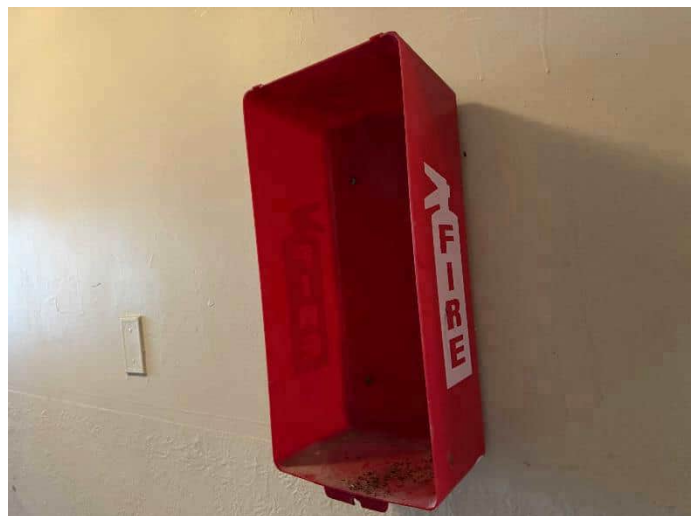
85. Building 2109 missing fire extinguisher.
