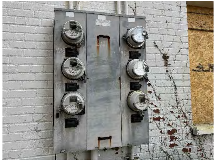
75. Utility meter bank.
