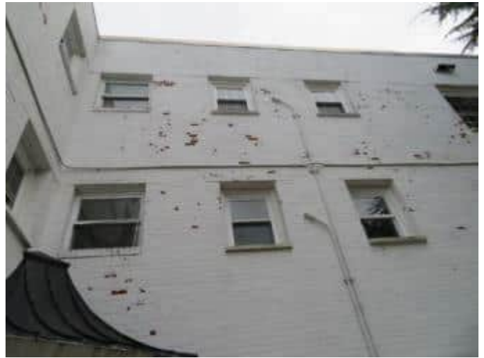
39. Areas of blistered and peeling paint at exterior.
