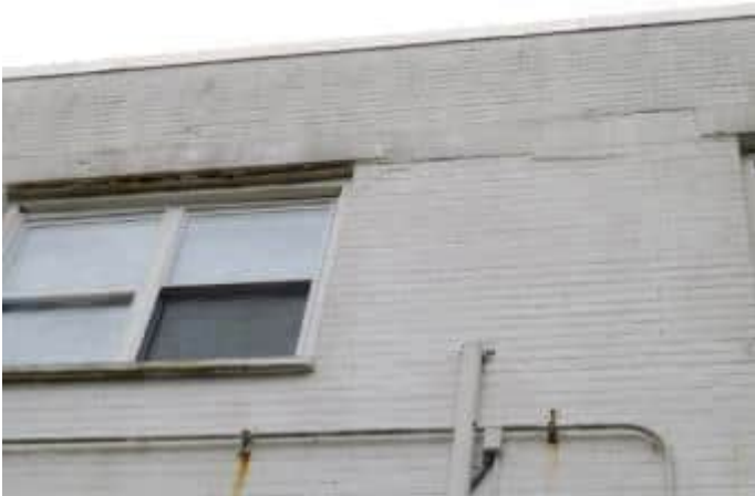
34. Evidence of possible off-plane movement over window unit.
