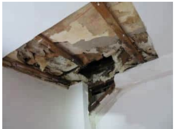
103. Water-damaged ceiling finishes and possible microbial growth.
