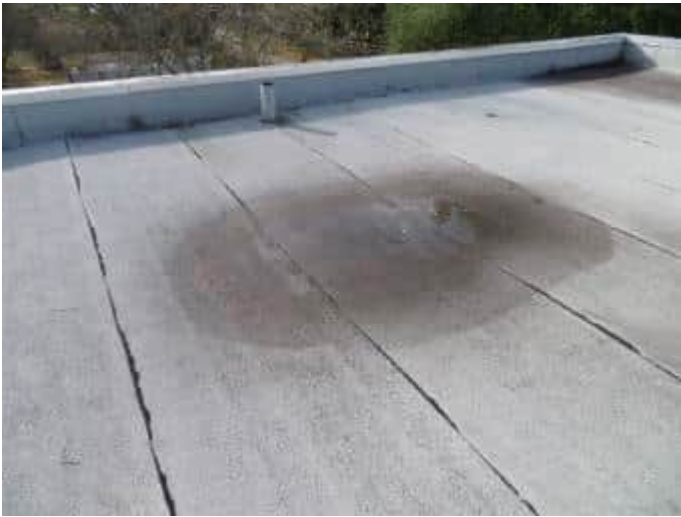
50. Localized area of possible ponding at built-up roof assembly.
