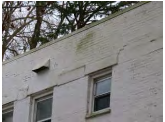
33. Possible off-plane movement at concrete over window.
