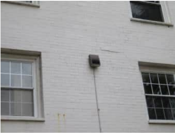
32. Localized cracking and possible off-plane movement.
